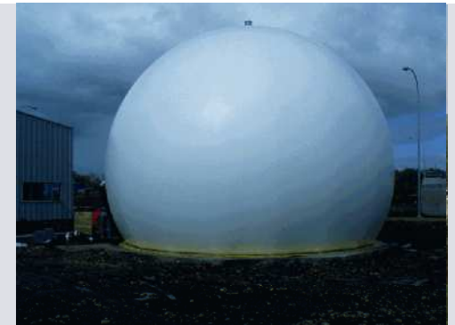
Wastewater Treatment / Volume: 590 m 3
