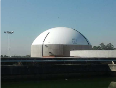
Wastewater Treatment / Volume: 2,040 m 3
