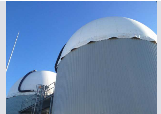
Composting Plant / Volume: 2 x 260 m 3
