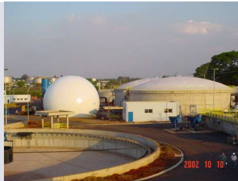
Wastewater Treatment / Volume: 2,250 m 3
