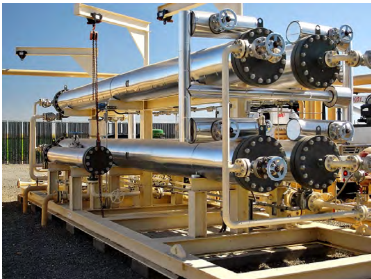
MTR supplied N 2 removal system operating in California
