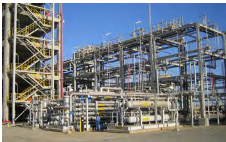
MTR supplied propylene recovery system operating in Middle East
